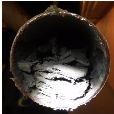
Pipes with amalgam sludge
